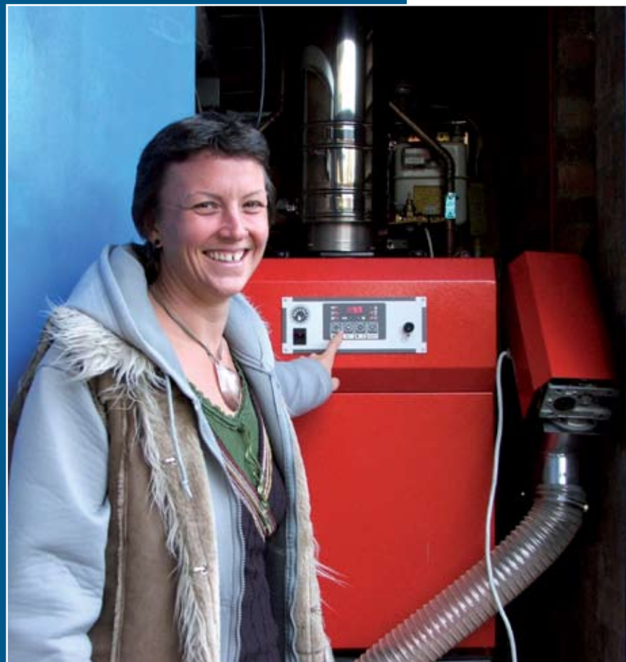
Gail Bamford of Sanford Housing Co-operative with the biomass boiler that has helped reduce their CO 2 emissions by 60%
